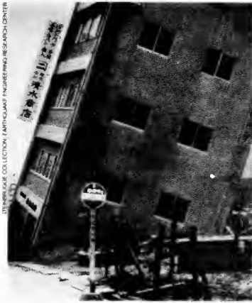
Failure of the ground itself can make an otherwise sound building unusable
