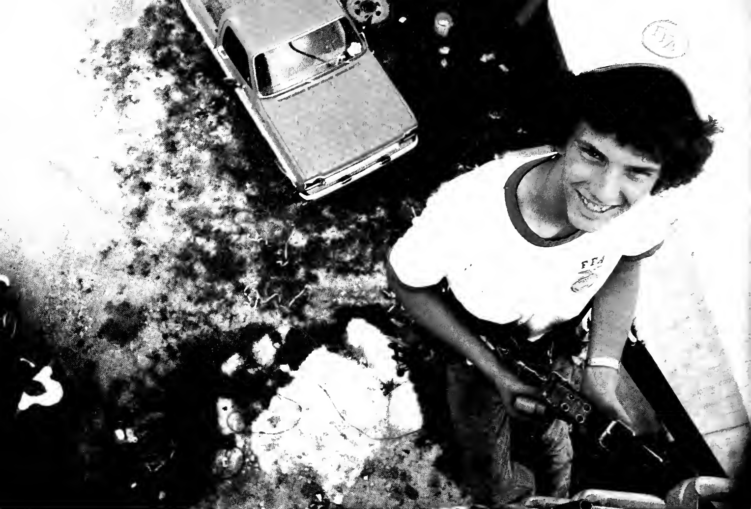
Mark's duties take him to soaring heights, exemplified here during a silo repair job.
