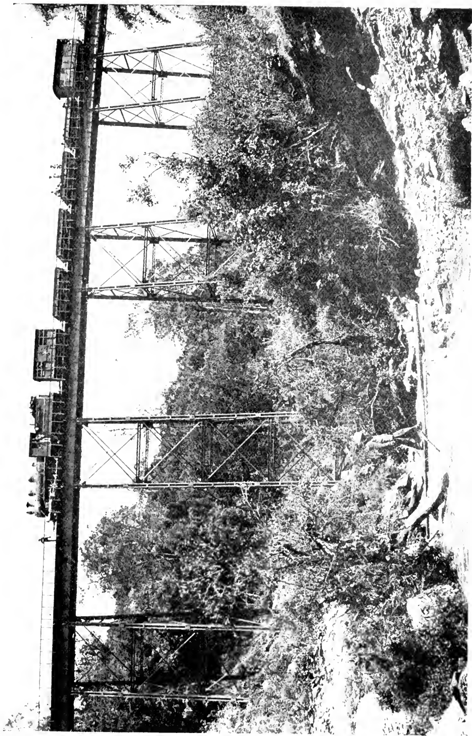
A BALDWIN LOCOMOTIVE ON AN AMERICAN BUILT VIADUCT ON THE MAU ESCARPMENT
