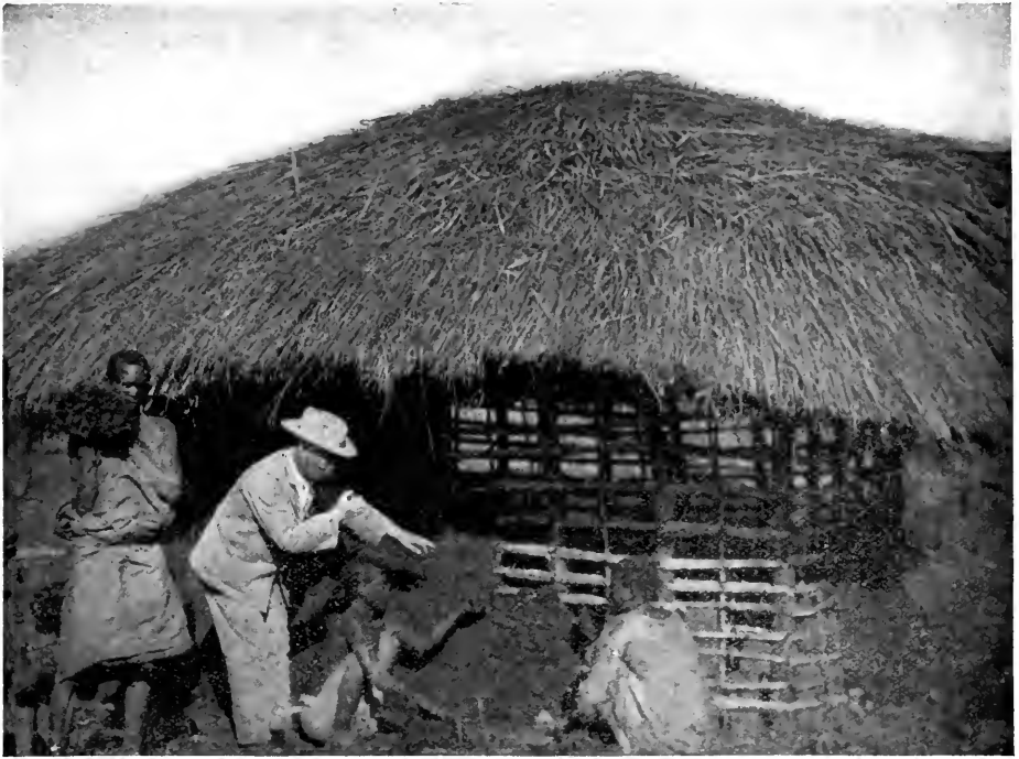
ARCHDEACON BUCKLEY, C. M. S., TEACHING BUSOGA NATIVES TO BUILD, DAUB AND WATTLE HOUSES
