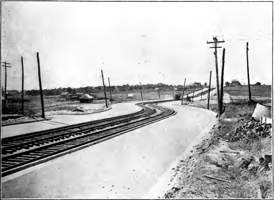
TRACK COMPLETED AND READY FOR BALLAST Oklahoma Railway Company, showing type of heavy track construction
