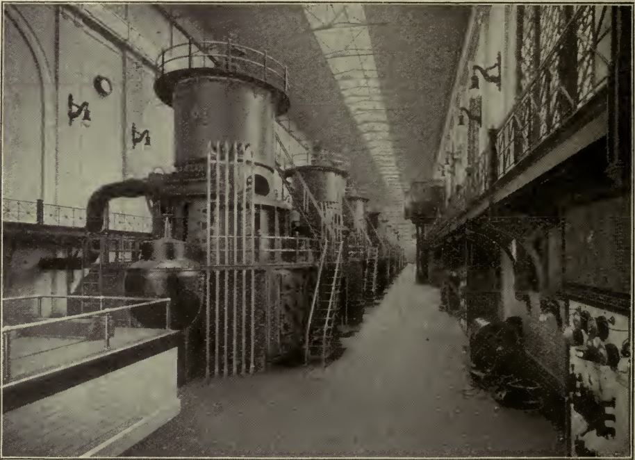
INTERIOR TURBINE ROOM, FISK STREET POWER HOUSE Ten steam Turbo-generators
