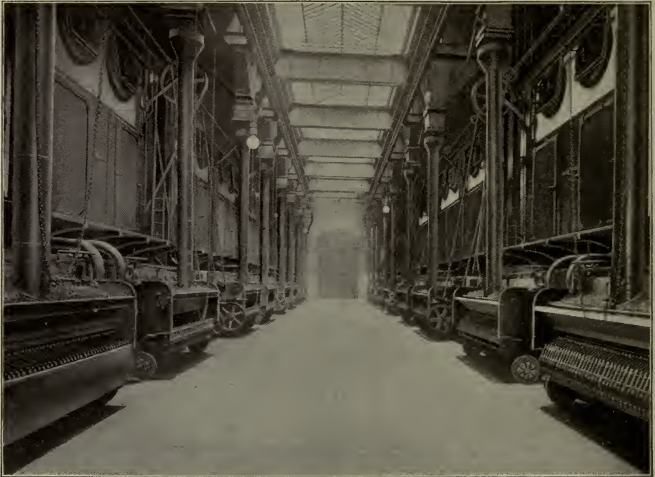
ONE BOILER ROOM SECTION OF THE FISK STREET STATION of the Commonwealth Edison Company. This section supplies steam for one Turbine
