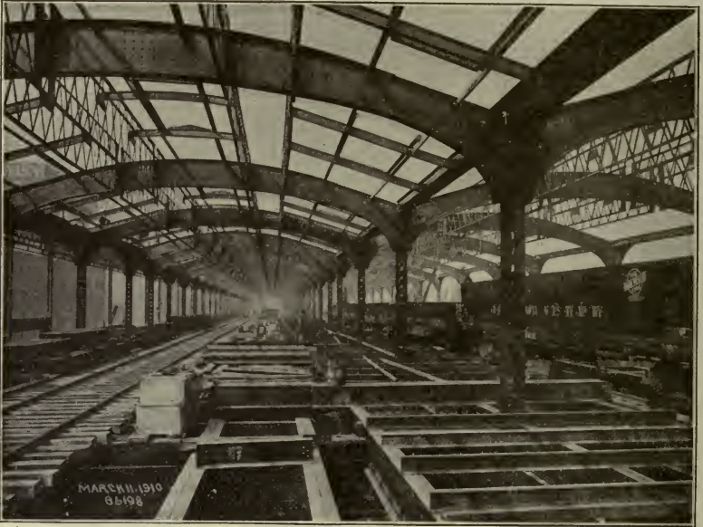
VIEW OF A PORTION OF THE CHICAGO & NORTHWESTERN NEW STATION IN CHICAGO
