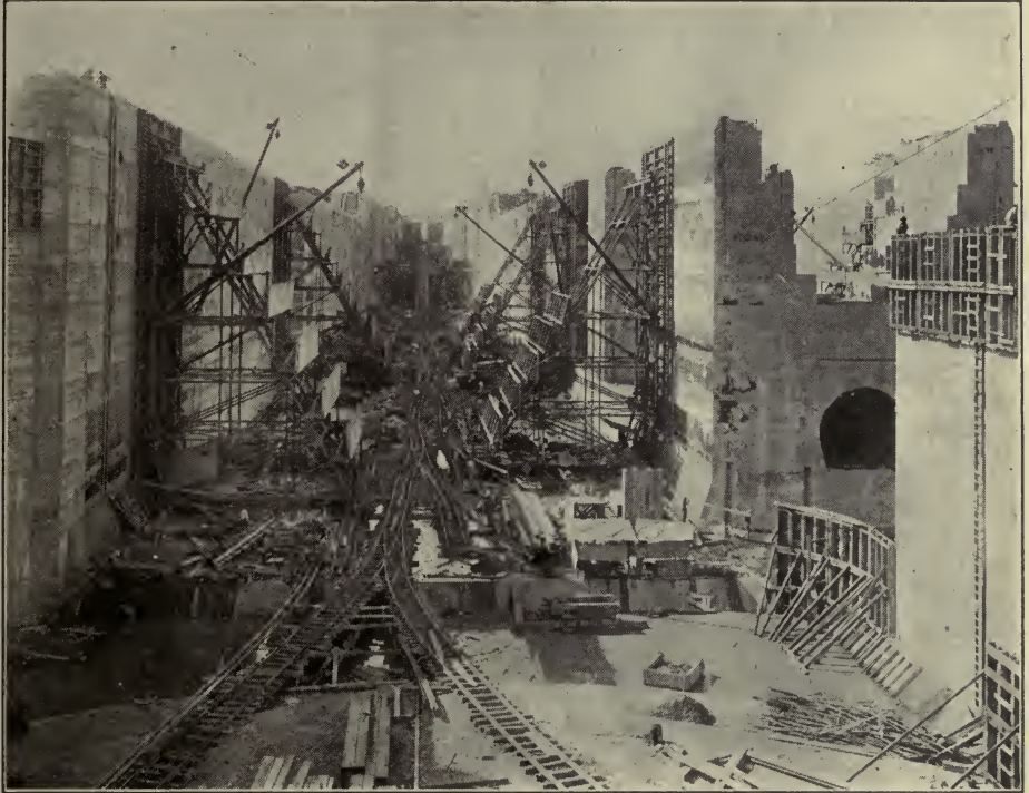
GATUN LOWER LOCKS, EAST CHAMBER, LOOKING SOUTH FROM COFFER-DAM, MIDDLE AND UPPER LOCKS IN DISTANCE
