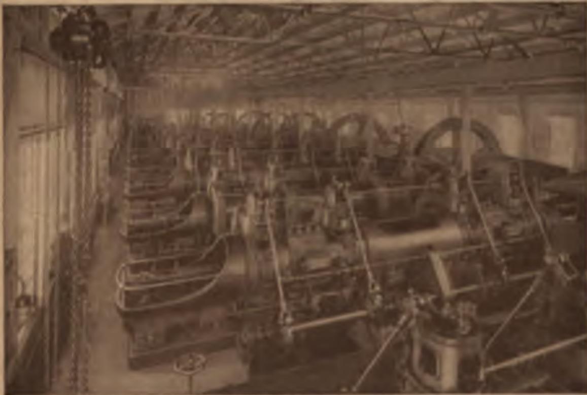
4500 H. P. of Cooper Gas Engine Driven Compressor Units in the Spencer, W. Va. Station of the United Fuel Gas Company.
