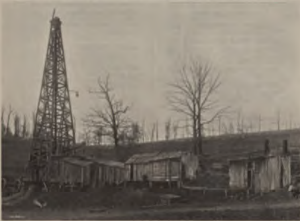
Well No. 4180 being drilled by the Hope Natural Gas Co. on the Mary Gull farm near Clarksburg, W. Va. On Jan. 29, 1918, the depth was 7,363 feet.
