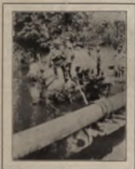
GAS LINE RESTING ON STONE.
