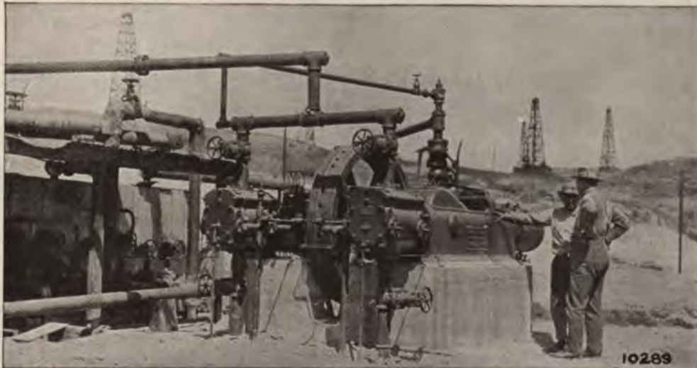
"Imperial" Type XPV Piston Valve Gas Expander recently installed at the Sunset Co.'s Plant
