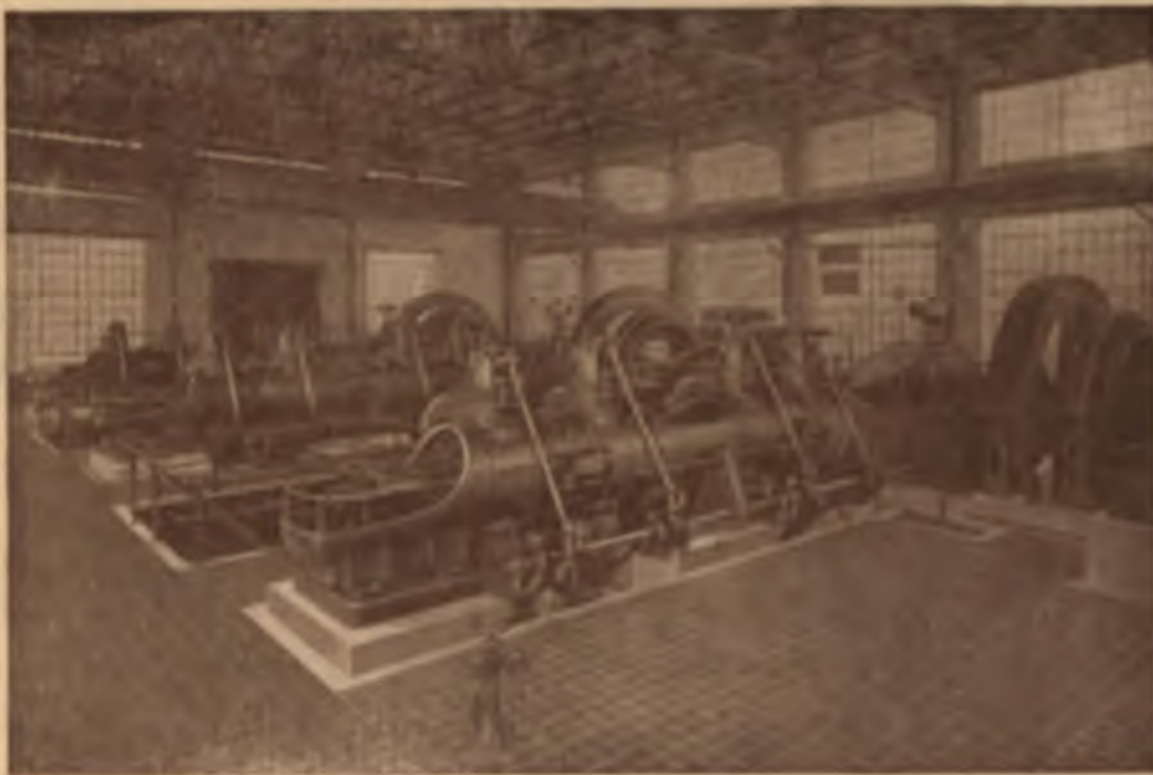
THREE 550 H. P. COOPER GAS ENGINES IN THE POWER PLANT OF THE LIBBEY-OWENS SHEET GLASS CO., CHARLESTON, W. VA.
