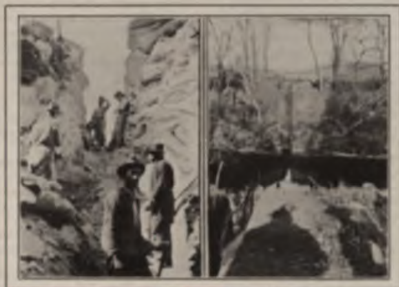
CUT FOR BLACKWELL LINE AT SILVER CREEK. SITE OF WALNUT RIVER CROSSING IN SOUTHERN KANSAS.
