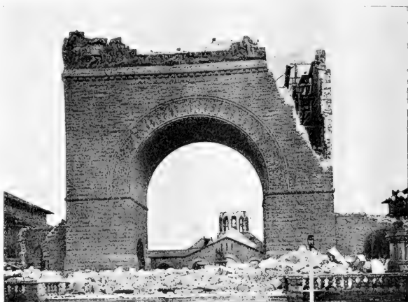
FIG. 2.—Memorial Arch, Leland Stanford Junior University. Earthquake Effect:—The beams designed to stiffen the walls were not tied to them, and helped to batter them down when the shock came. (Photograph by Richard L. Humphrey.)
