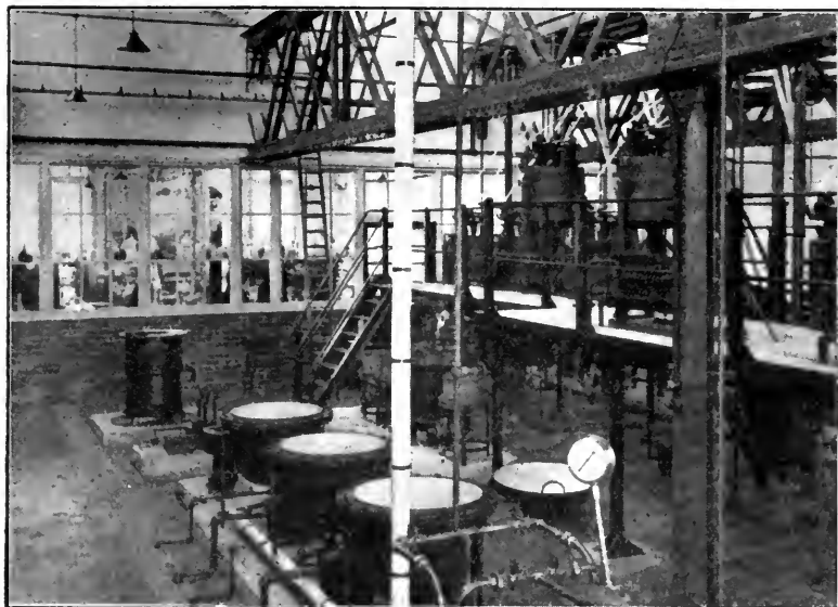
FIG. 2.—View towards S.E. showing evaporating pans, centrifuges, and box filters. Research laboratory through screen.
