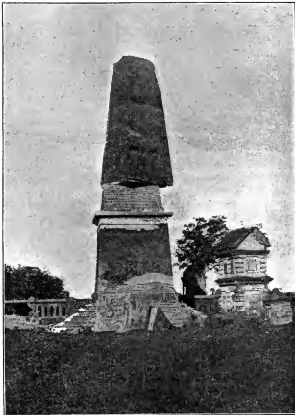
FIG. 1.—Monument at Chhatak, with part twisted by earthquake. The part of the monument left standing is about 46 feet high.
