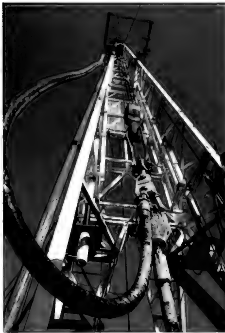
A towering drill rig holds the enormous drill shaft in a vertical position so it can penetrate deep into the earth.
