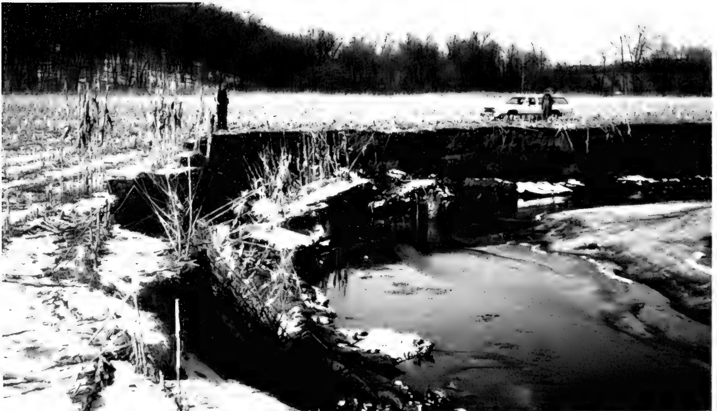
Two rows of corn are shown washed into the stream channel of Court Creek in February 1986.
