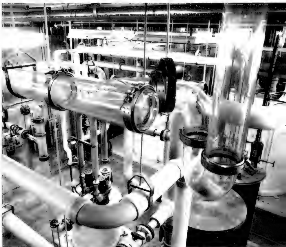
Maze of large diameter Pyrex glass piping safely conducts potentially hazardous lab wastes to a series of sedimentation and holding tanks.
