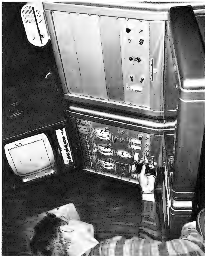
Figure 3. Control instrumentation for DOTIPOS components.
