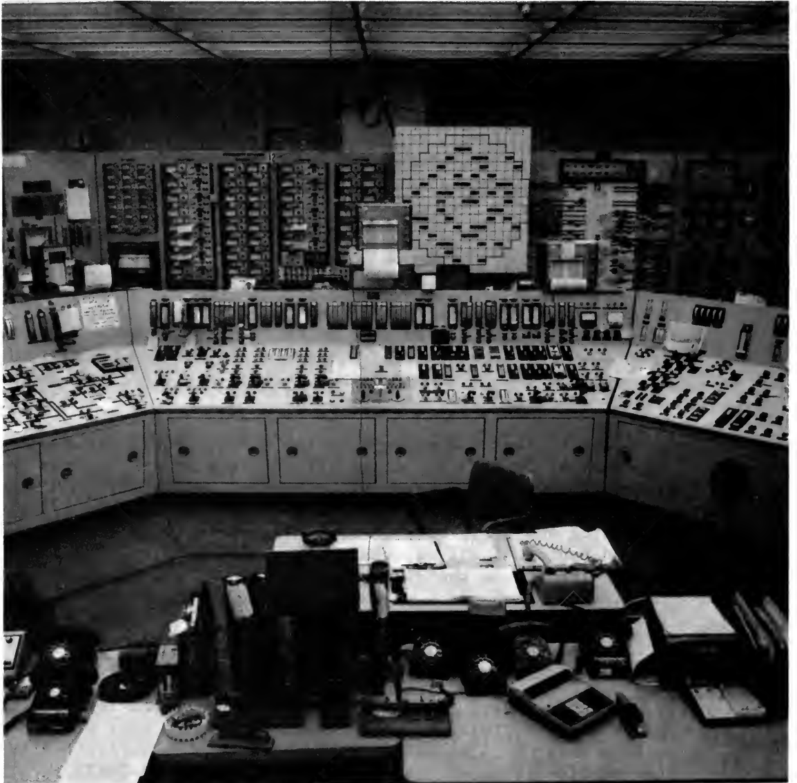
TMI-2 control room.
