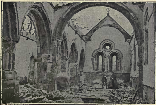
SHERBURN HOSPITAL CHAPEL. Interior after the last fire. (See p. 183.)
