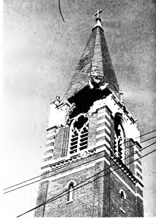
Northeast of Yantic, JEWETT CITY saw its imposing brick church put up a valiant fight against the hurricane. Twice the steeple appeared ready to go. A low-flying plane might have smashed that gaping hole in the belfry. The hole widened under terrific pressure. Miraculously, the steeple stayed aloft.
