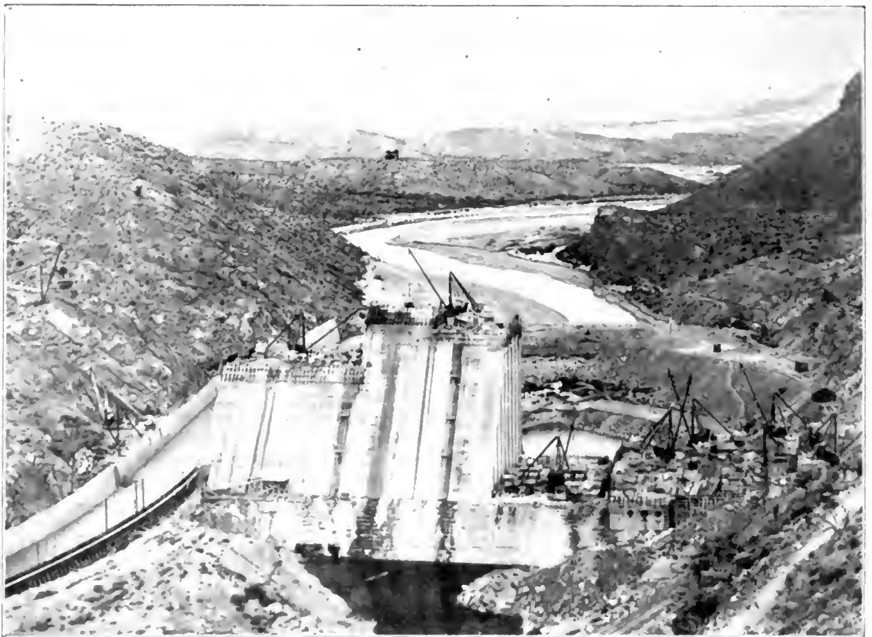
ELEPHANT BUTTE DAM SITE LOOKING NORTH FROM EAST BANK - NOTE SLUICE TUNNEL GATES AND LANDING PLATFORM
