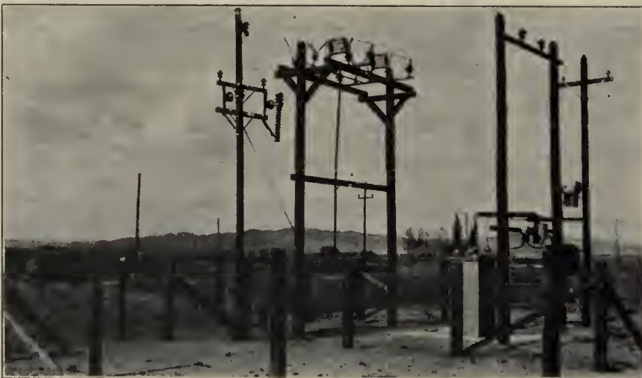
Single-phase substation, electric power system, Truckee-Carson irrigation district
