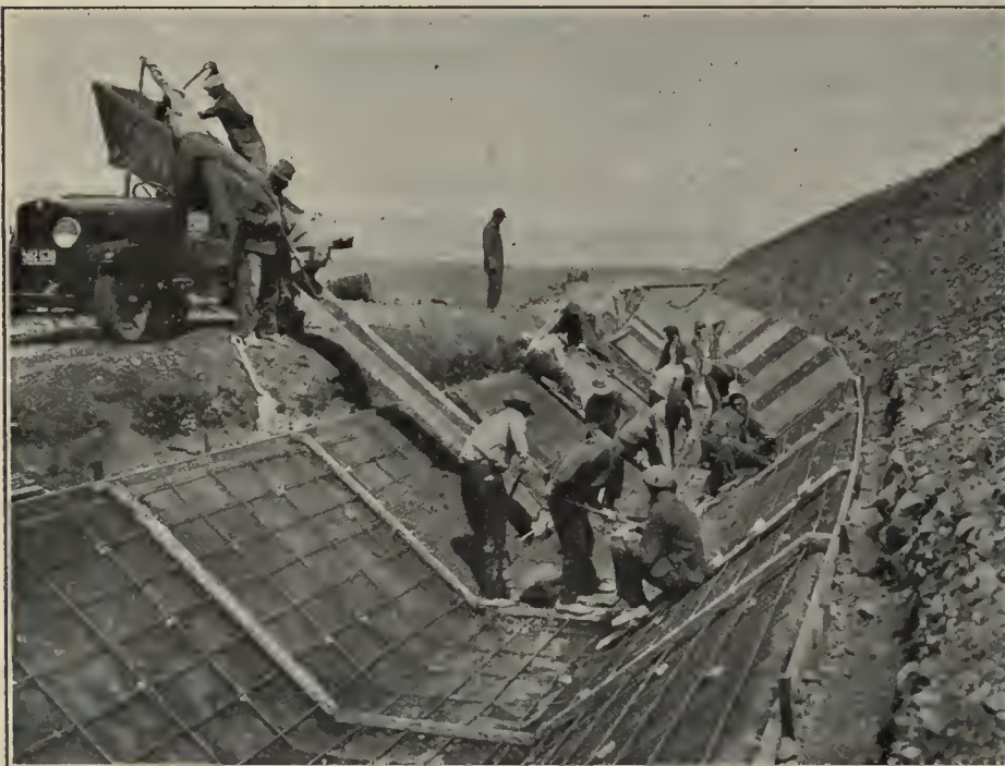
Concrete canal lining (concrete placed by hand), South Branch Canal, Kittitas division, Yakima project, Washington
