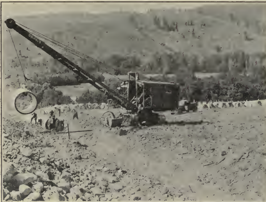
Dragline handling 54-inch lock-joint pipe, South Branch Canal, Kittitas division, Yakima project, Washington
