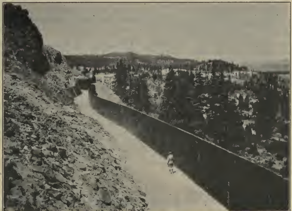
Combination section of Kittitas Main Canal, near Morrison Canyon, Yakima project, Washington
