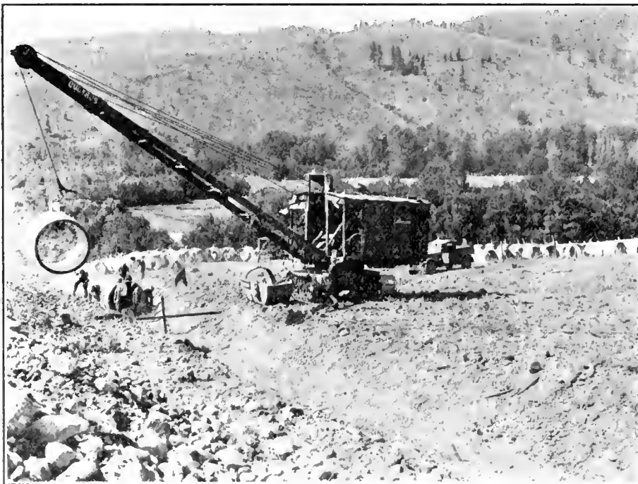
Dragline handling 54-inch lock-joint pipe, South Branch Canal, Kittitas division, Yakima project, Washington
