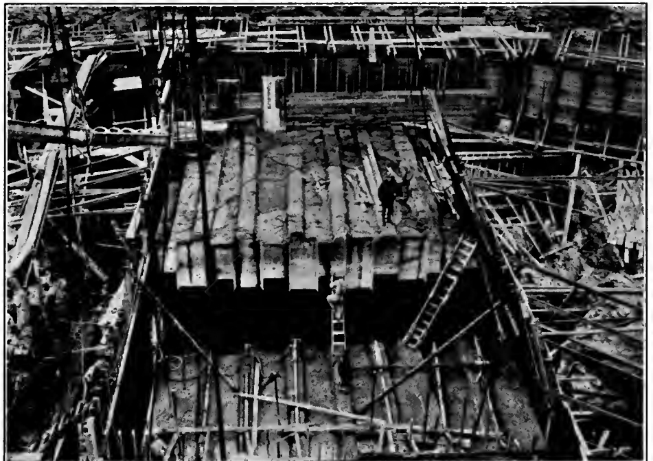
Construction progress at Easton diversion dam, Kittitas division, Yakima project, Wash., looking toward north abutment, showing concrete placed in spillway section
