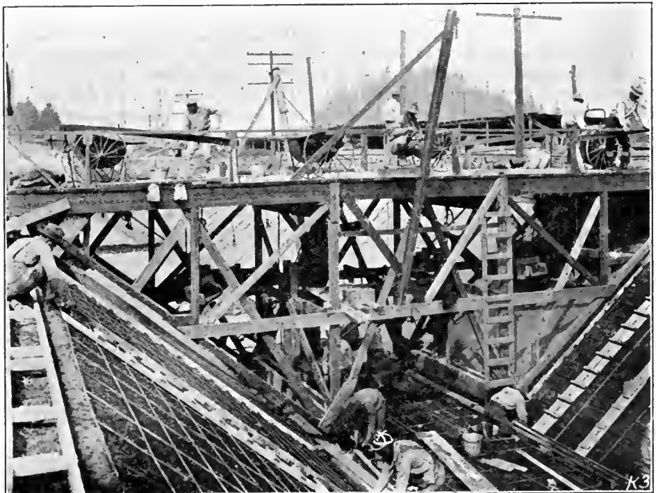
Apparatus used in placing concrete canal lining, Kittitas Main Canal, Kittitas division, Yakima project, Washington
