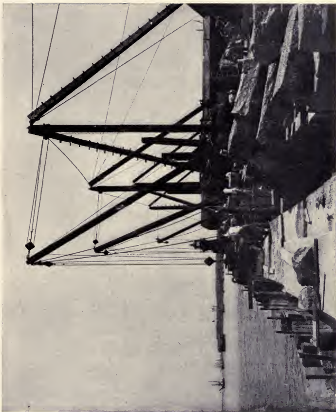
"THE SEA WALL THAT BABCOCK WAS BUILDING FOR THE LIGHTHOUSE DEPARTMENT." — F. HOPKINSON SMITH'S "TOM Grogan."
