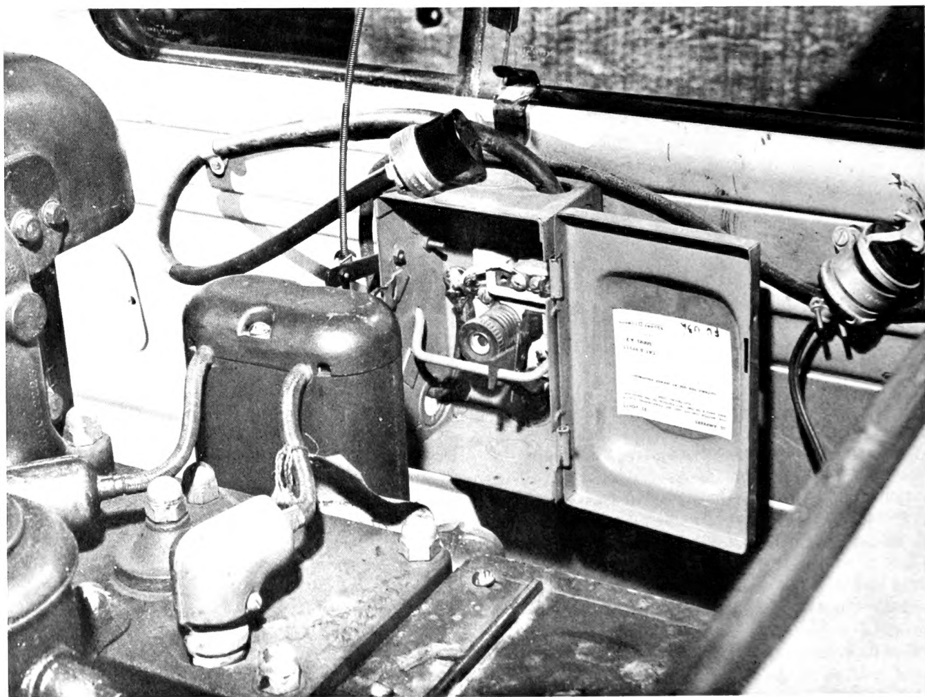
Fig. 4.—The 110-volt switch box, with fuse, mounted on the wall of the truck alongside the generator. The electrical cable that enters the switch box at the lower left corner is the lead from the 110-volt power outlet of the generator. The electrical cable that leaves the switch box at the upper right corner terminates in a female receptacle that connects with a cable from the floodlight cluster. The flexible control cable is shown attached to the circuit-breaker arm of the switch box. The receptacle and plug for the hand-held spotlight are shown connected at the far right.
