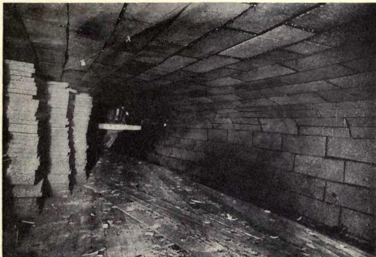
Nonpareil Corkboard erected in asphalt cement and nailed in place in the hold of the famous clipper ship, "Glory of the Seas," now turned into a floating cold storage plant. Notice how the corkboard has been fitted to the irregular wall surfaces.
