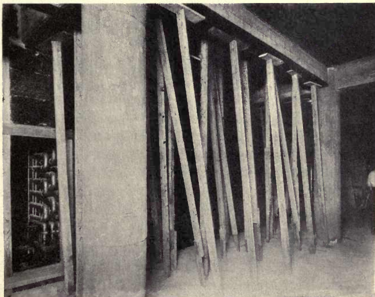
In erecting Nonpareil Corkboard against concrete ceilings, the boards are coated with Portland cement mortar and propped in place until the cement sets. This view was taken at the St. Louis Refrigerating & Cold Storage Company's plant, St. Louis, Mo.
