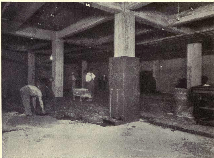
Installing Nonpareil Corkboard on floor and columns. Terminal Freezing & Heating Company, Baltimore, Md.
