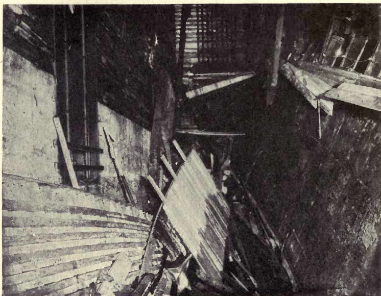
Boards-and-air-space insulation, rotted out after only six years' service in a Philadelphia cold storage plant
