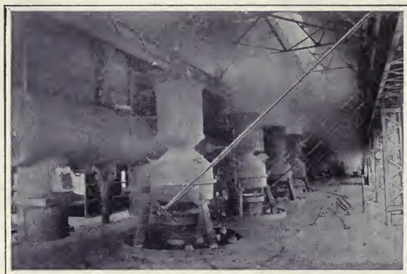
CHARGING FLOOR OF THE BATTERY OF GAS PRODUCERS SHOWING ROCKING ARMS FOR GRADUAL FEEDING OF THE COAL
