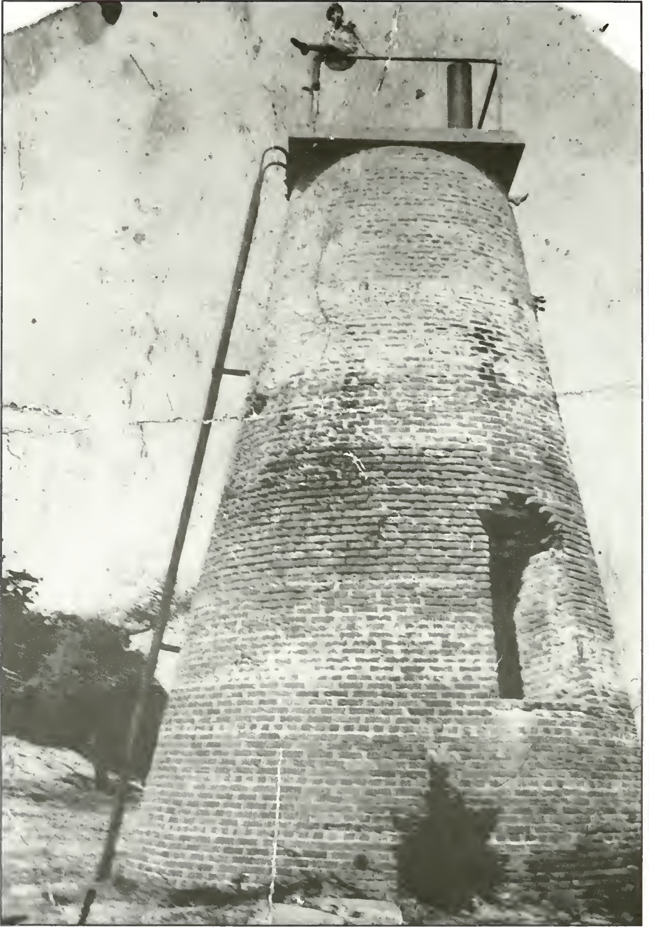
Civil War cannon damage at the base of the Price's Creek Lighthouse. (N. C. Division of Archives and History photograph)
