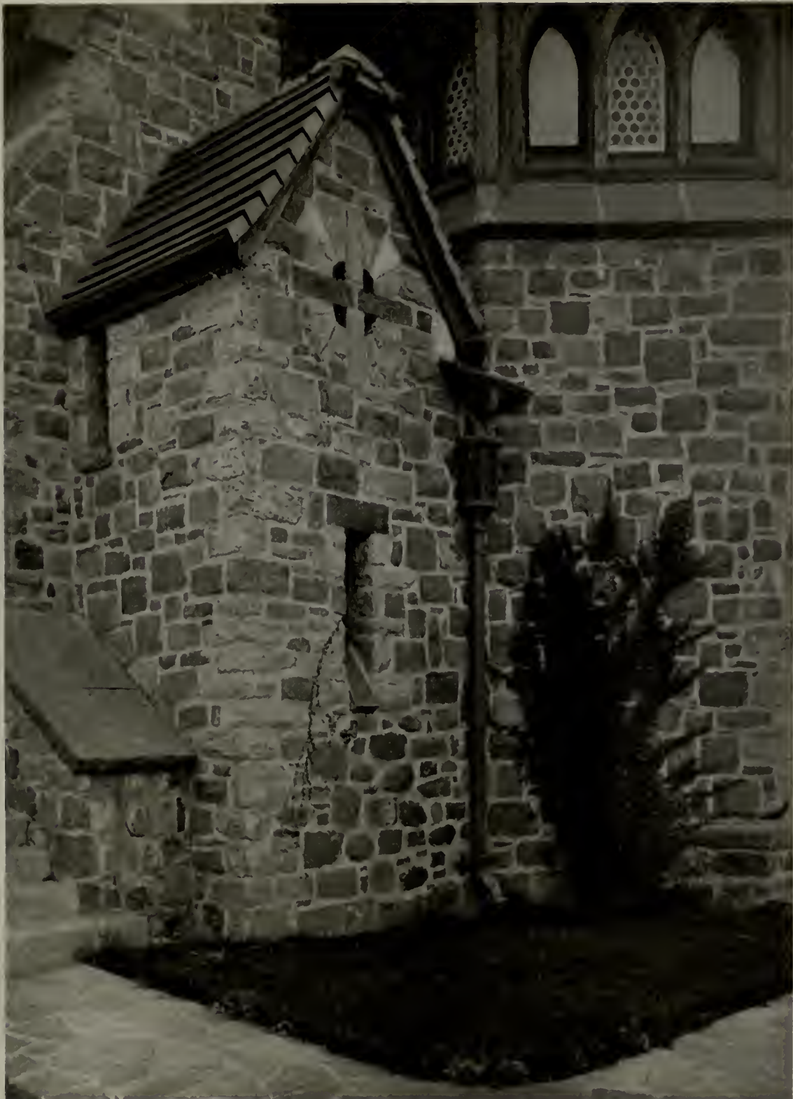
DETAIL OF THE EAST END THE CHURCH IN THE GARDENS, FOREST HILLS, N. Y. GROSVENOR ATTERBURY, ARCHITECT
