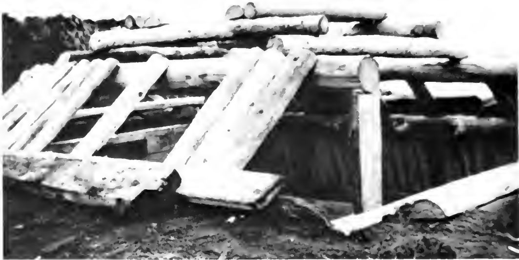
FIG. 62. Partially constructed house roof. There are four support posts, one of which is visible, on which rests a four-layer cribbing of horizontal logs. Walls are of vertical split logs and roof two courses of slanting split logs (one unfinished course shown).
