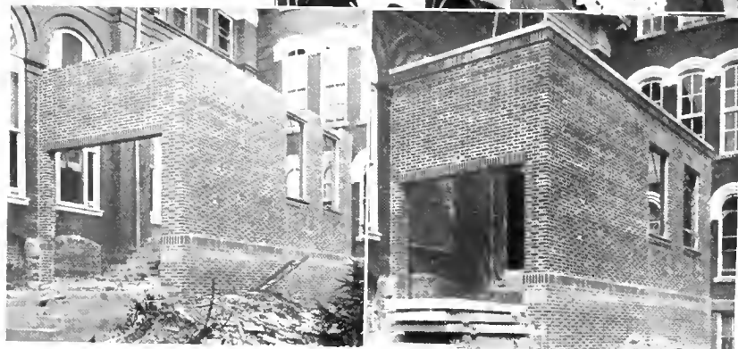
After. The first and last opening of the locked fire escape.
