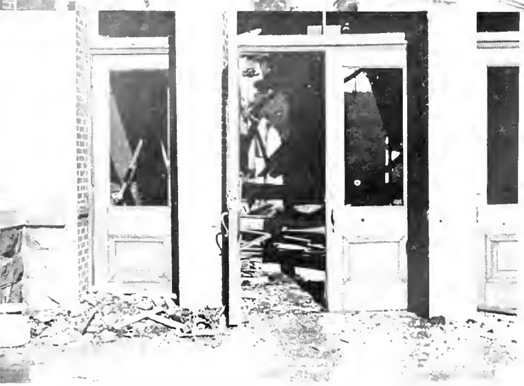
Aftermath of the fire in old Leonard Hall.
