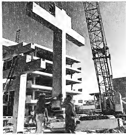
Construction continued on the three-stage building complex for the School of Technology.
