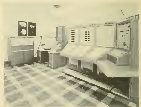
FIGURE 6-7. Prototype central control station showing displays and computer. Manufactured by Westinghouse Air Arm.
