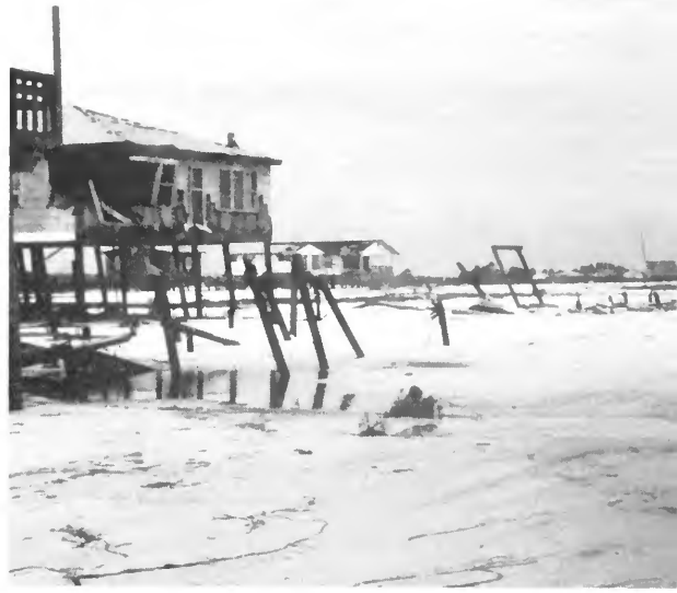
Pilings leaning before the wind are dramatic, if mute, evidence of the wind and wave forces of Hurricane Frederic. Inadequate piling depths, liquefied sand, poor piling-to-floor connections, and inadequate pile bracing contributed to the failures of these houses during the storm.
