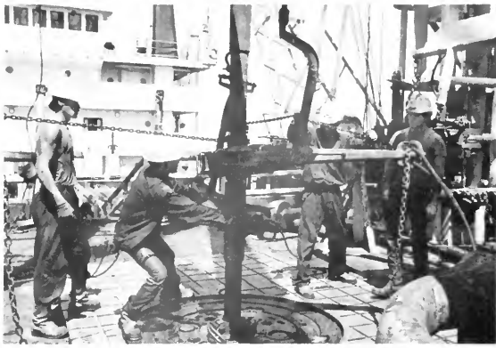
Chinese and American roustabouts at work on the Java Sea, a drill ship that works the South China Sea. (Huang Jianqiu/HNA)
