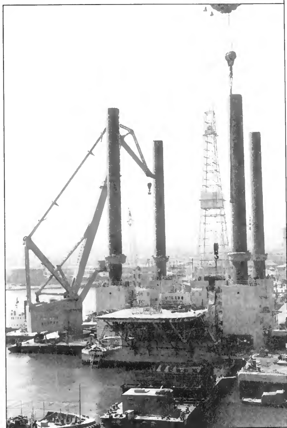
A marine oil-drilling derrick being built at the Dalian Shipyard in Northeast China. (Eastfoto)
