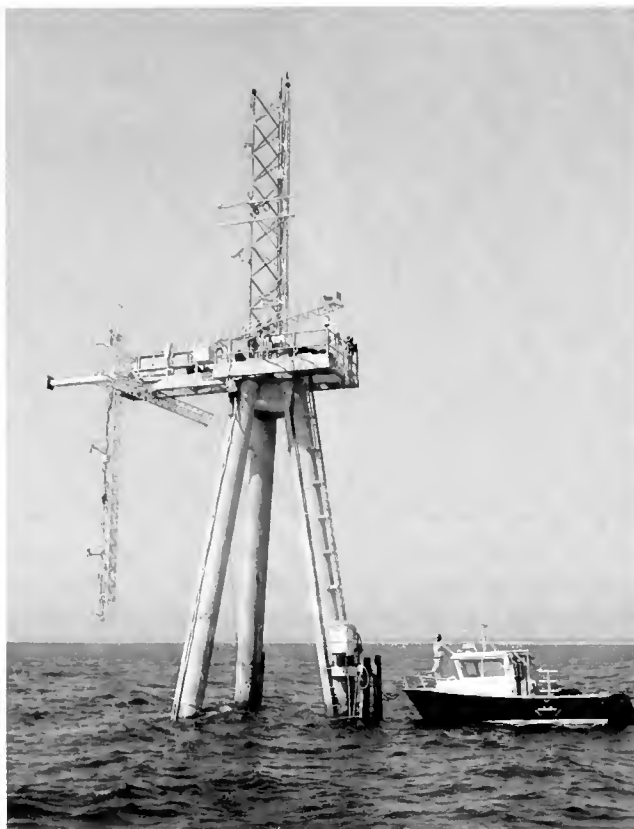
STANDING TALL—The Air-Sea Interaction Tower, built as part of an experiment sponsored by the Office of Naval Research, allows scientists to deploy instruments that monitor the relationship between winds and waves in all weather conditions.
