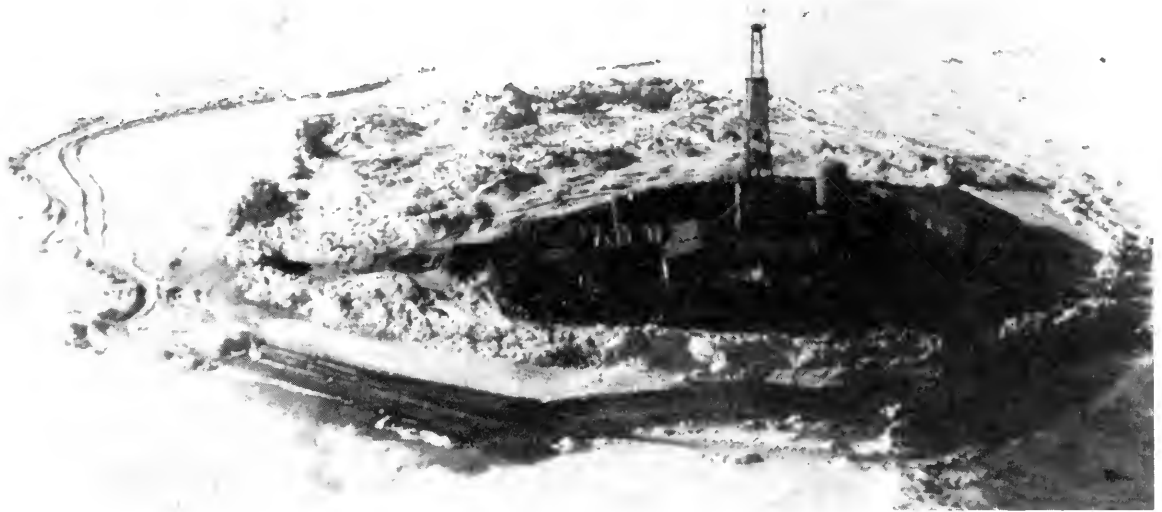
Figure 4. Drilling operations from an artificial island during winter. (Photo courtesy of Canadian Marine Drilling, Ltd.)
