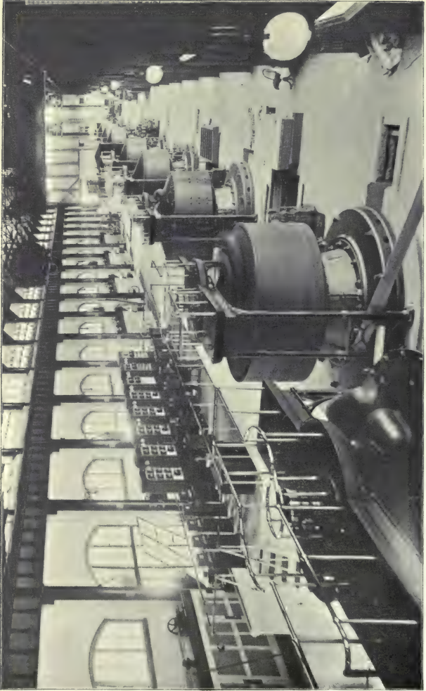
INTERIOR OF THE POWER HOUSE.
