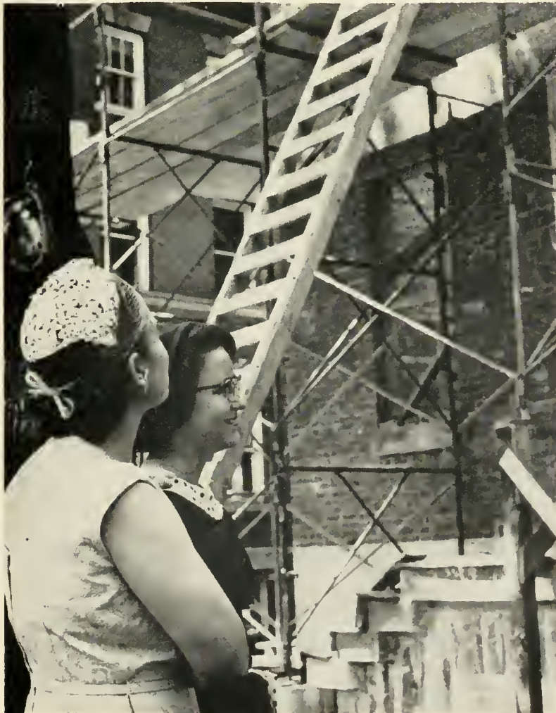
TOUR OF CAMPUS gives mom a chance to see changes which are taking place. Here she and Anito inspect progress of Helen Mauck Galbreath Memorial Chapel.
