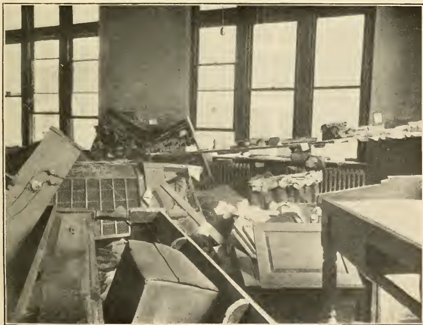
.B. POST OFFICE, DAYTON, OHIO, AFTER THE FLOOD OF MARCH-APRIL, 1913.
