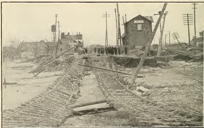
B. RAILROAD CROSSING AT SOUTH HAMILTON, OHIO, AFTER THE FLOOD OF MARCH-APRIL, 1913.
