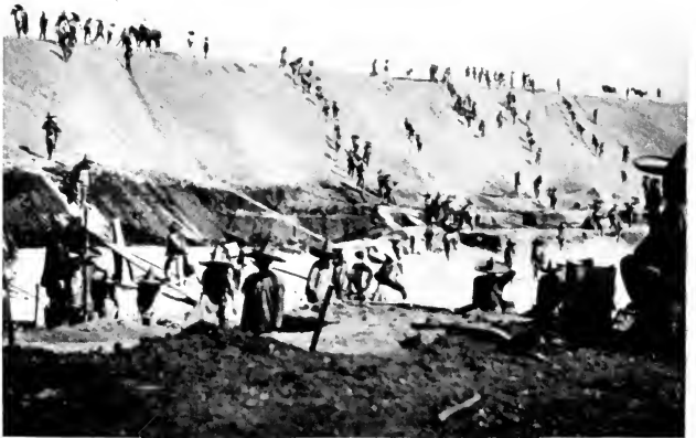
BUILDING THE EARTH RESERVOIR TO RECEIVE THE FLOW FROM POTRERO DE LLANO NO. 4.
