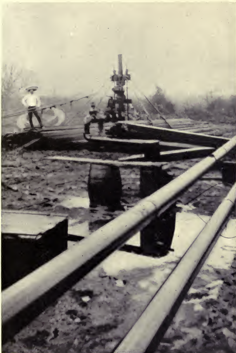
THE GATE VALVE WHEREWITH THE MEXICAN GUSHER POTRERO DE LLANO NO. 4 WAS BROUGHT UNDER CONTROL.
