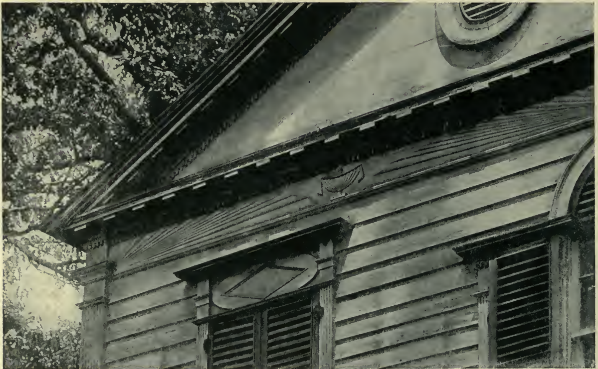
Detail of Entablature and Window Head. HOUSE AT CHATHAM CENTER, NEW YORK.
