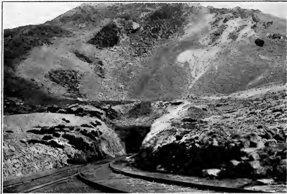
GALERA TUNNEL. HIGHEST POINT ON THE OROYA RAILWAY, NEARLY SEVENTEEN THOUSAND FEET ABOVE THE SEA.
