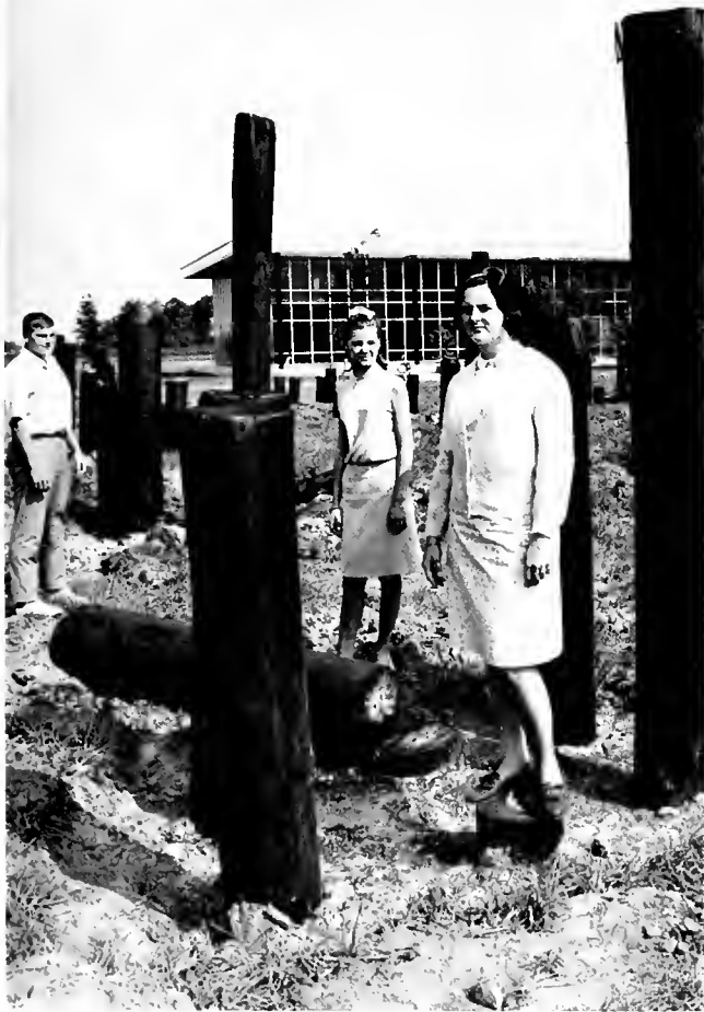
Clark Dail, Nancy Peacock, and Pam Thomas inspect the library construction which began at the start of the summer session.
