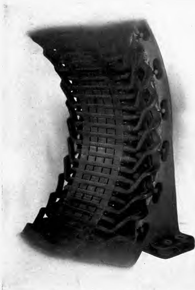
FIG. 8.—Armature Winding of 275 K.W., 600 R.P.M., 3 Phase, 60 Cycle Generator.
