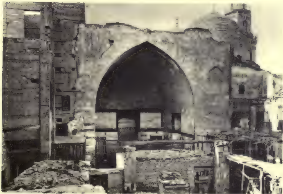
B. — Cairo : Madrasa of Sultan as-Sâlih Negm ad-Din Ayyûb — northern half, west liwân.
