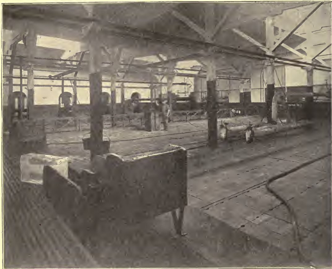
FREEZING TANK ROOM IN AN ICE FACTORY.
