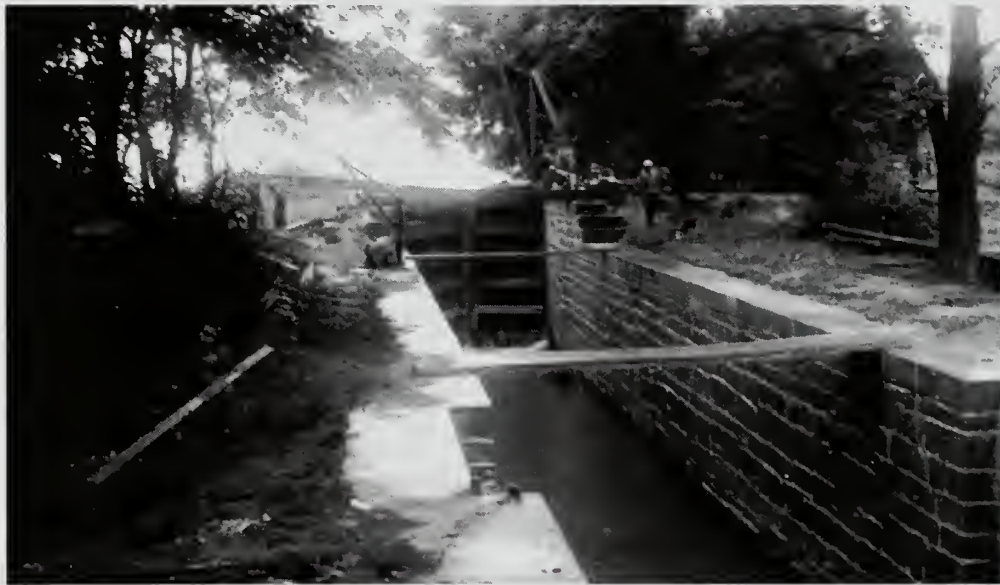
Photograph 19: Feeder Lock with inlet gate closed. The water entering the canal here serves all the way to Lock No. 5.
