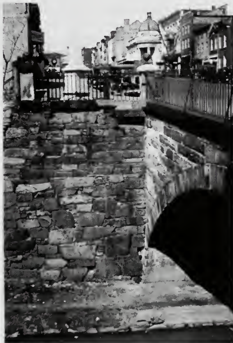
Photograph 5: Northwest corner of Wisconsin Avenue Bridge. Note character of masonry of bridge and retaining wall, the sturdy wrought iron fence, and the memorial obelisk.
