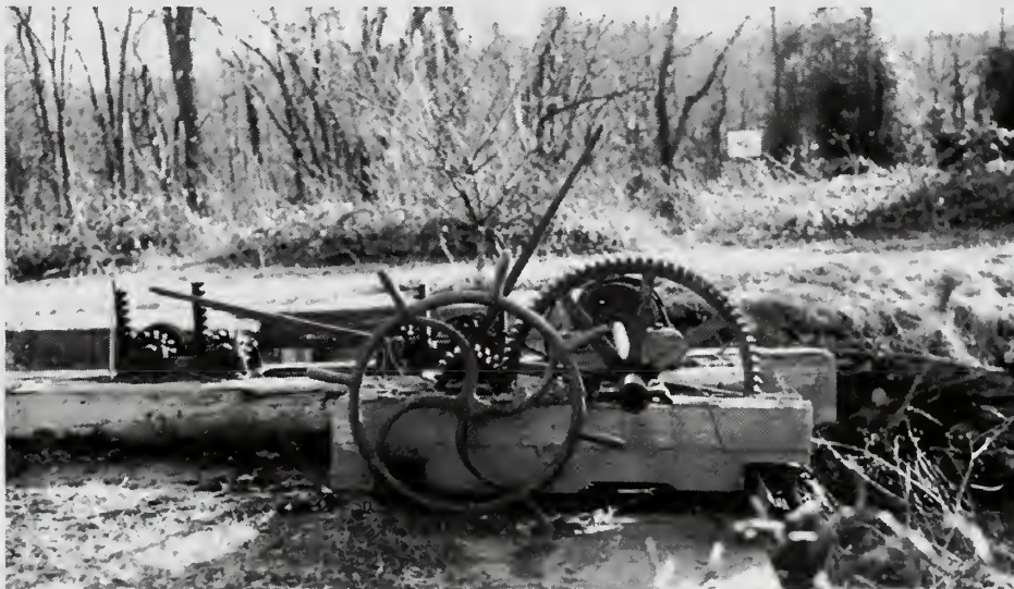
Photograph 3: Machinery for raising and lowering gate.
