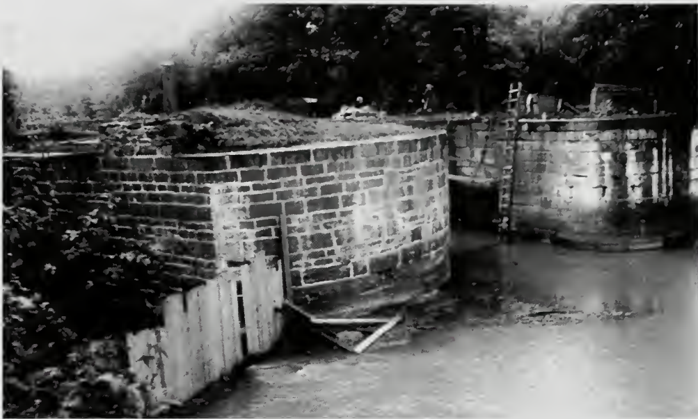
Photograph 18: Lock No. 23 at right, Feeder Lock at left. On Feeder Lock wall is a masonry abutment for the mule-crossing that carried the towpath.
