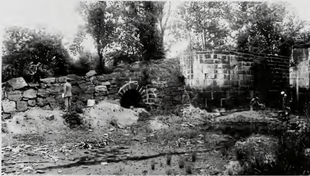
Photograph 14: Spillway culvert, south end of Lock No. 18, carrying excess water under the towpath to the River. This masonry has been repointed.
