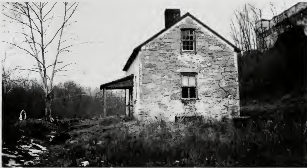
Photograph 29: House at Lock No. 7. Settlement cracks in the wall, carelessly rebuilt after the 1936 flood tore away some of it. This had to be taken down and relaid before the work of restoration for use could be carried out. Here again dormer windows and plumbing were added and the interior rearranged for greater economy and comfort.
