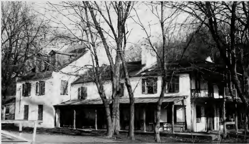
Photograph 45: Tavern from the southwest. Part of this brick addition of 1832 is in bad condition and repairs are to be made. This tavern has served its purpose almost continuously for more than a century, operated by the members of one family since the Civil War.
