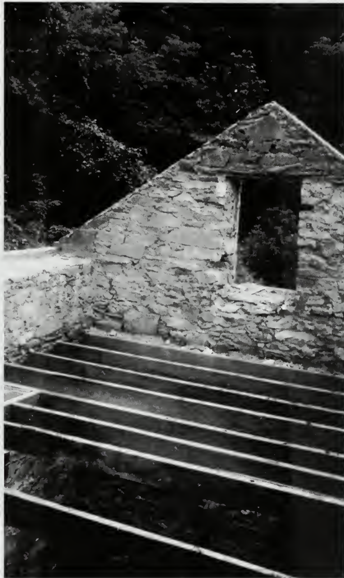
Photograph 30: The masonry of house at Lock No. 7. This shows the plate resting on the stone wall without the wooden grounds called for by the specifications; also the joists are built into the masonry.
