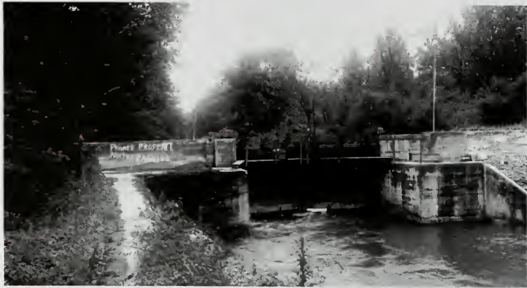
Photograph 16: Control Gate on Feeder Canal where it enters canal at Lock No. 5.
