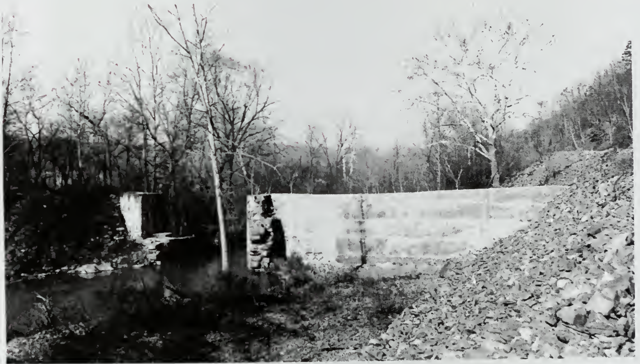
Photograph 20: Stop Lock above Lock No. 16, showing the abutments and the new concrete core wall covering the old masonry core at the Berm, or east end.
