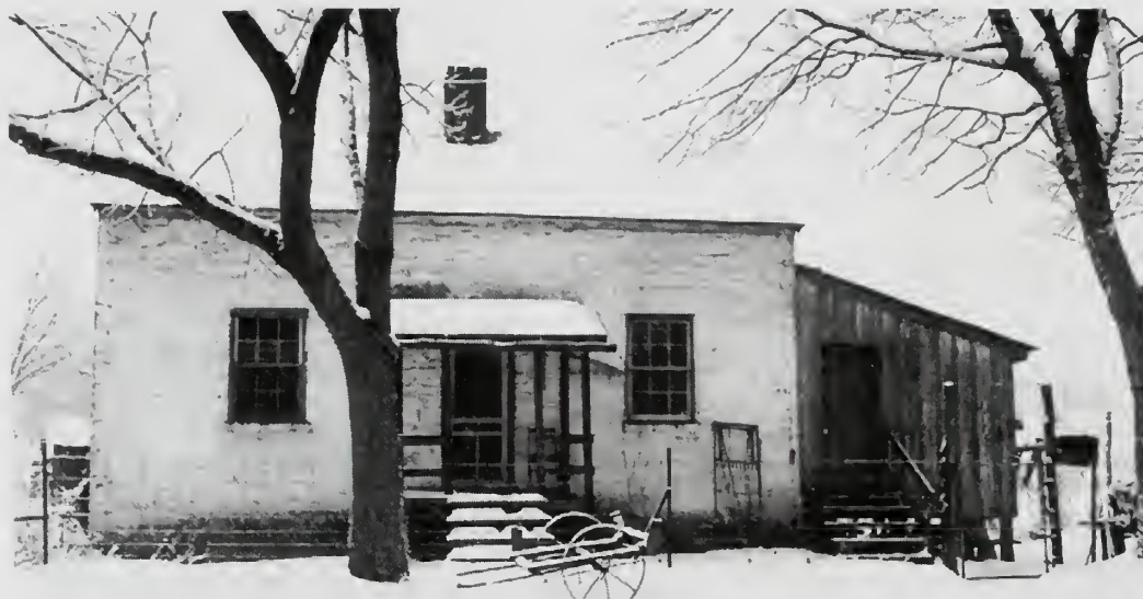
Photograph 35: House at Lock No. 11. This house on the towpath side has a small shed addition; it is in fair condition, and will continue in use as it is.
