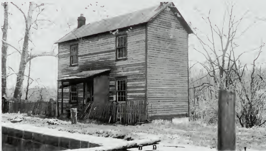
Photograph 38: House at Lock No. 14. A departure from type. Frame structure on the towpath side. Substantial repairs will be needed here if this house is to be used.
