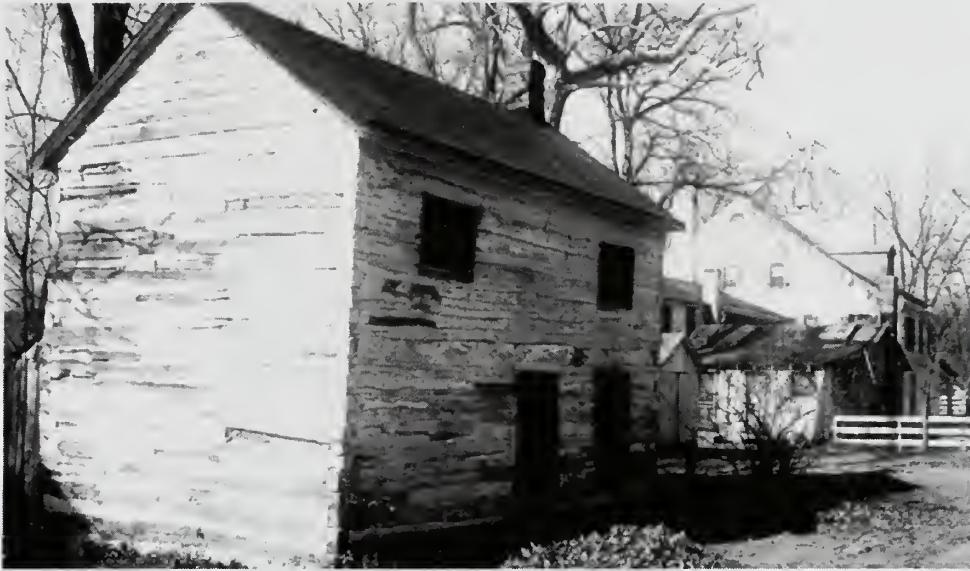
Photograph 47: The Log House south of Tavern, built of hewn logs about 1884. This is to be repaired for use as a Lock Tender's House. It is described by those who live in it as particularly cool in summer and warm in winter.
