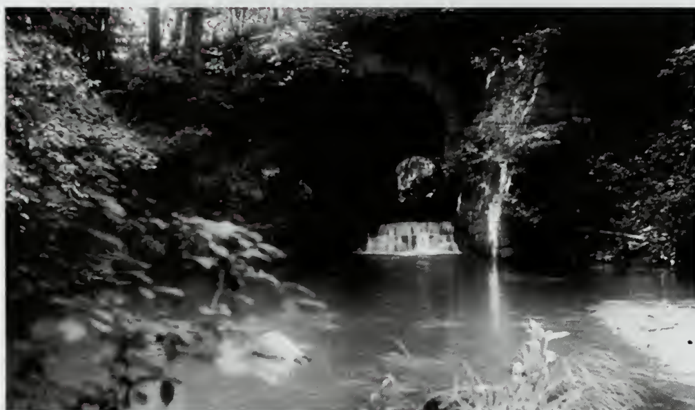
Photograph 13: Rock Run Culvert, below Lock No. 11. An excellent example of the substantial character and simple design of the canal masonry.
