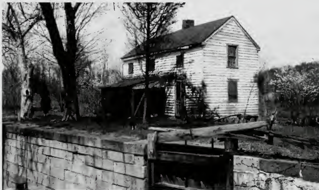
Photograph 36: House at Lock No. 12. A frame building differing from the established type. There are only shallow foundations, no cellar. If the building is to be used it virtually will have to be rebuilt. The lock wall appears in foreground.
