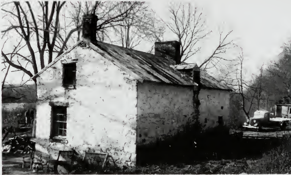
Photograph 51: House at Swain's Lock (No. 21). This building varies from the established type. Its relationship to the lock can be judged from the lock curbing in the left foreground. The structure is in fair condition and continues in use.
