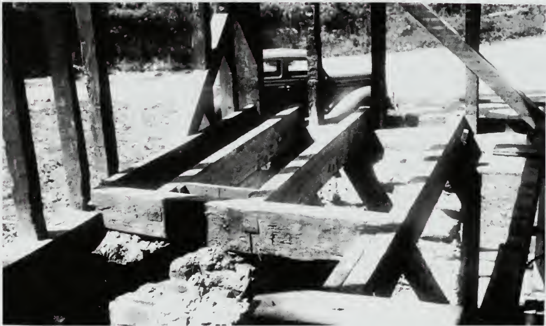
Photograph 27: Another view of the old framing; the header at the hearth, showing tail joints mortised and pegged. This framing is found to be generally in sound condition although it has stood since 1853, when this house was rebuilt. With very little repair it is serving now.
