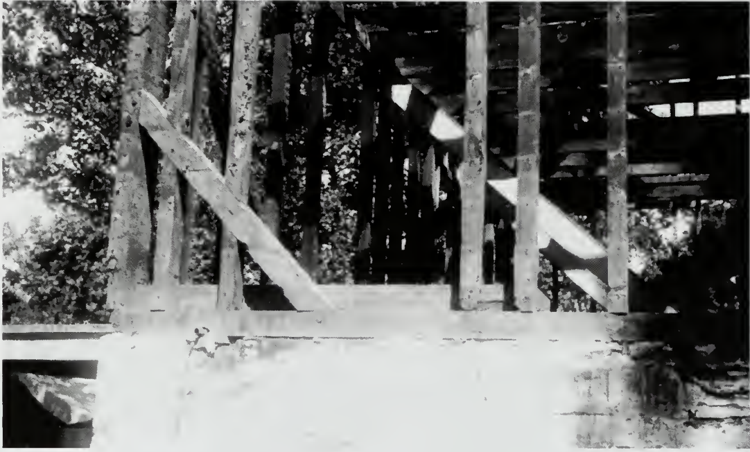
Photograph 26: The framing of the house at Lock No. 5. The diagonal braces were mortised and pegged into both the posts and the sills. Note that rats have gnawed away the studding just above the sill.
