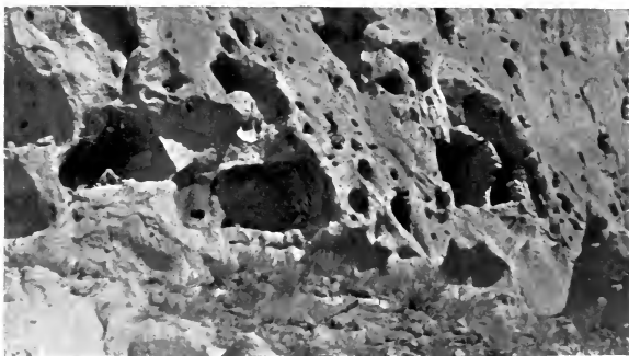
Mausard-Collier Eng. Co. CAVES AND EROSION IN THE CLIFF.
