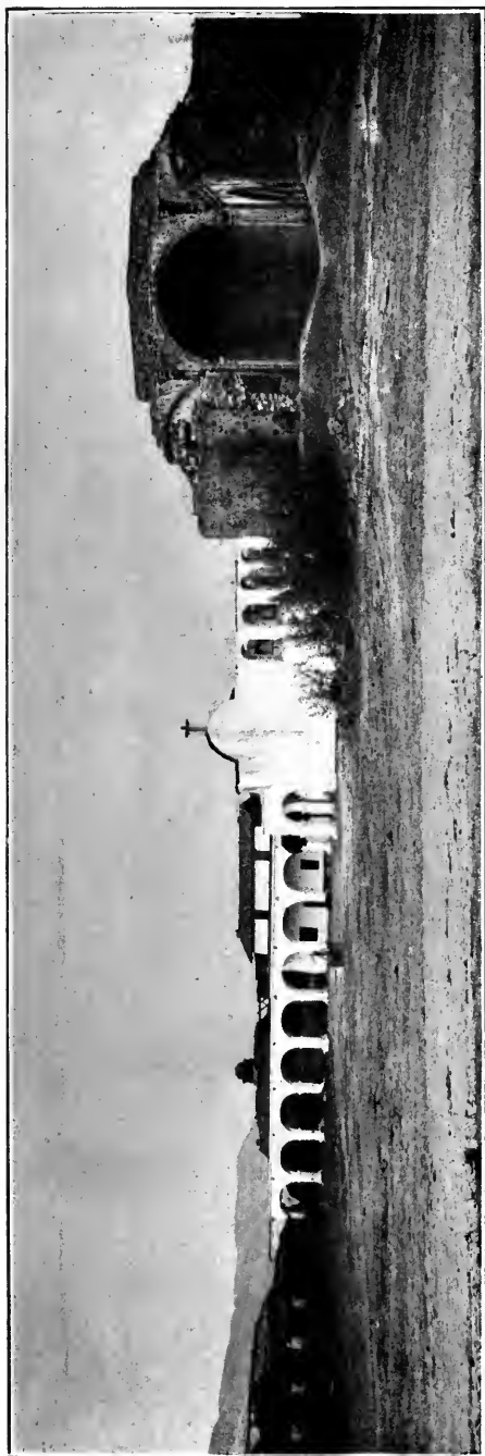
FRONT OF SAN JUAN CAPISTRANO. (Shows broken roofs, debris in stone church, etc.)
