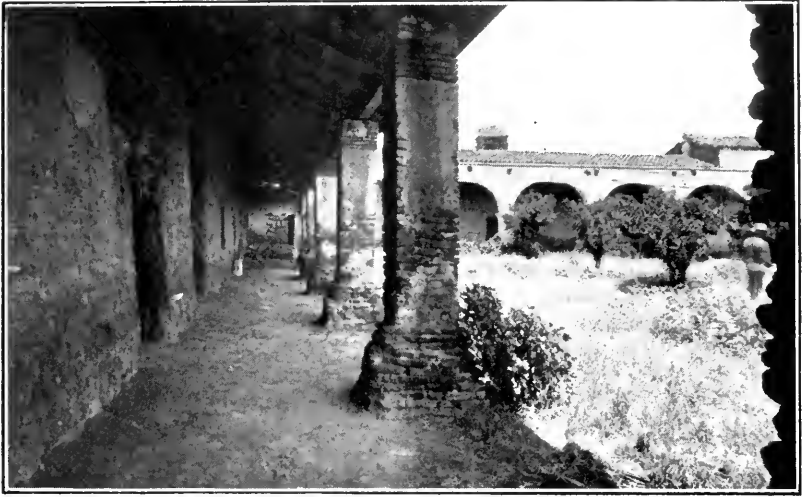
CAPISTRANO—in corridor of building Photo by C. F. L., June 4, 1903 just reroofed by the Club.
