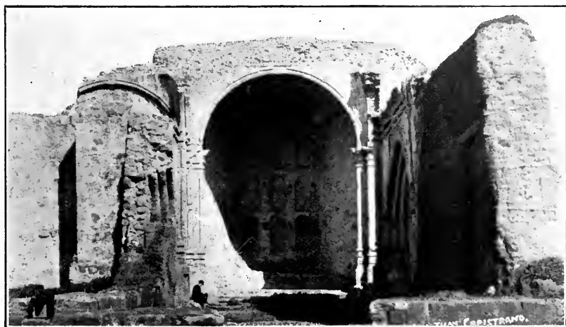
CAPISTRANO—Remains of the great stone church. Debris removed by the Club. See cut on p. 7.
