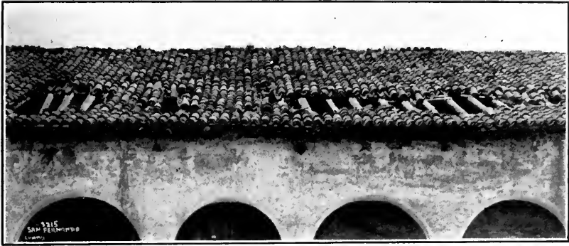
SAN FERNANDO MISSION. Photoby C. F. L., 1800 [Condition'of the Monastery roof (70 x 240 ft.) before the Club's work.
