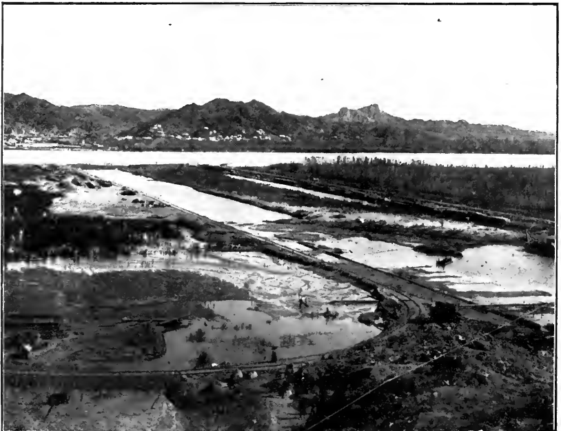
GENERAL VIEW OF LAGUNA DAM FROM CALIFORNIA SIDE, SHOWING GOVERNMENT AND CONTRACTOR'S CAMP.
