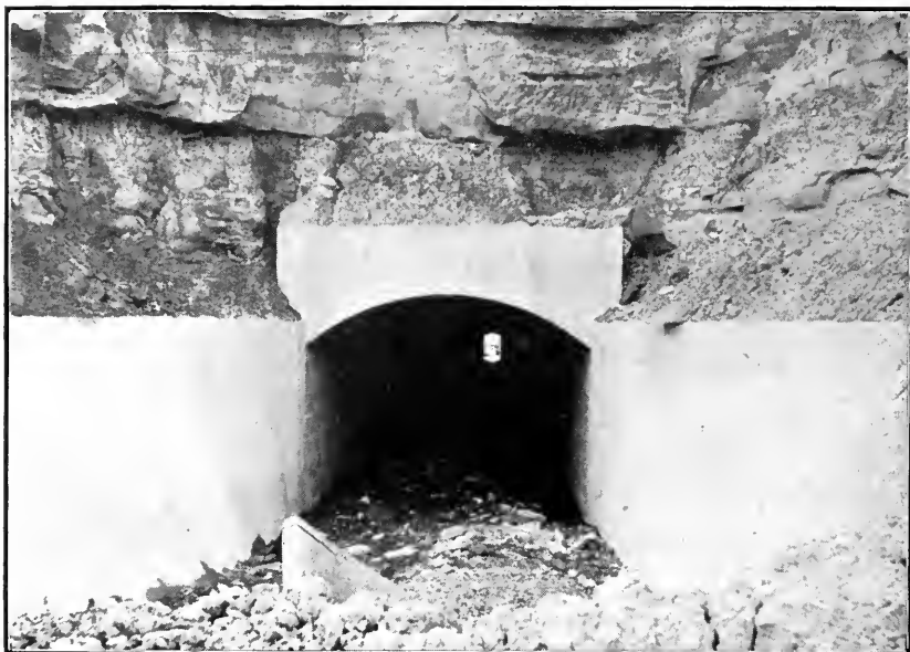
PORTAL TO TUNNEL, ON DITCH. There are about fifteen of these in all.
