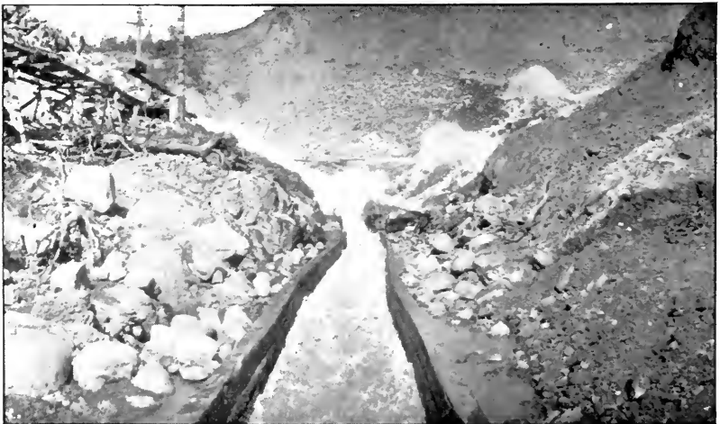
SLUICE-BOXES WITH FULL PIPE HEAD
